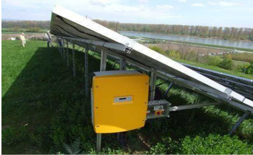
Fig 1.23: solar inverter (yellow) mounted to the solar racking converts DC electricity from the solar array to useful AC electricity
