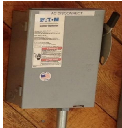
Figure 1.22. Examples of AC safety disconnect switch boxes.
