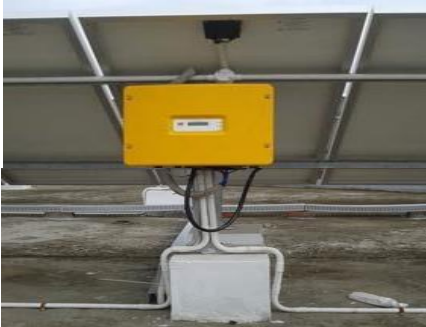
Fig 1.6: Field Junction Box (FJB)
